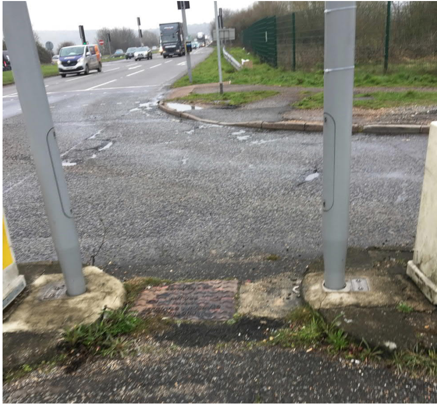
Figure 19 – Footway surface opposite Old Shoreham Road at the Sussex Pad junction looking east.
